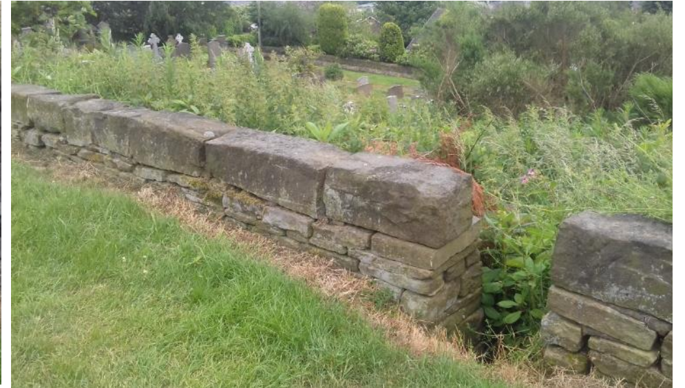
Photo 9: Gap in wall onto 'Moss Side' half way between point A and point E 22/6/2017
